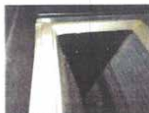
View of Coil Chamber
